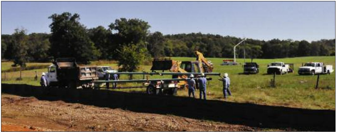
FPU gas, water and electric construction crews work together to build utility services into the Douglas-Posey Industrial Park along Highway 64 East.
